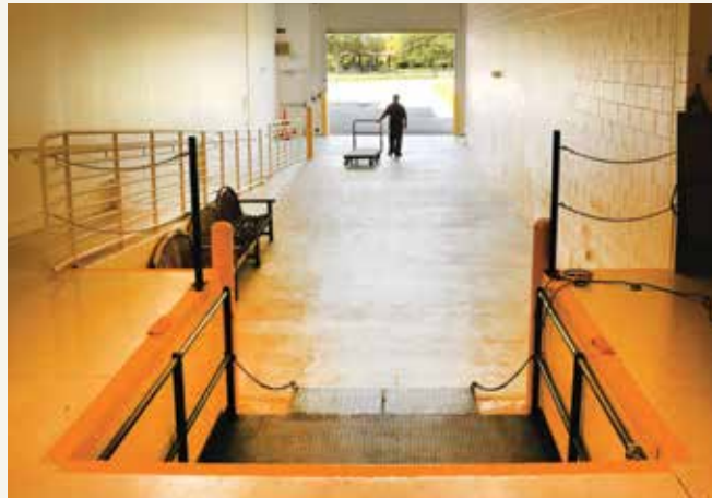
After the garage door closes, the temperature and humidity will be brought up to match the conditions inside a climate-controlled truck.
